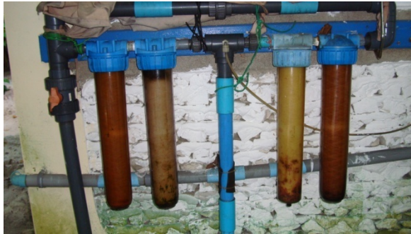
Figure 5-2: Micron filters of the first plant are installed outside the plant building
