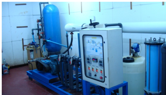
Figure 5-1: The second plant of 50m 3 /day showing the plant room is kept dry and well maintained
