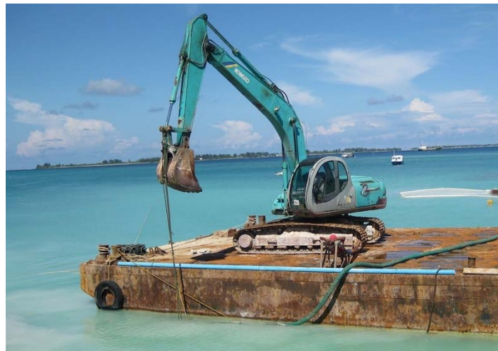
Figure 1: An excavator mounted on barge will be used to deploy the concrete footings at the site.
